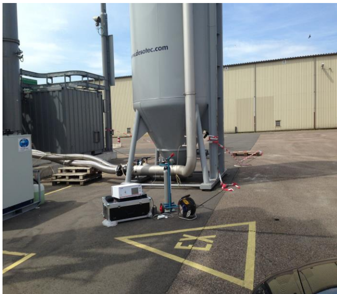
Figure 7: GC-IMS SILOX on-site. The instrument precisely quantifies individual siloxanes species, L2-L5 same as D3-D5, calculates 'total silicon' and 'total silica' and by this allows to take a reliable decision on-site. Besides a flexible spot-to-spot measurement using its one-click operation it even enables a continuous and remote online monitoring to test for the pipe gas same as for a potential filter breakthrough while sampling and quantifying the siloxanes automatically in user defined intervals.
